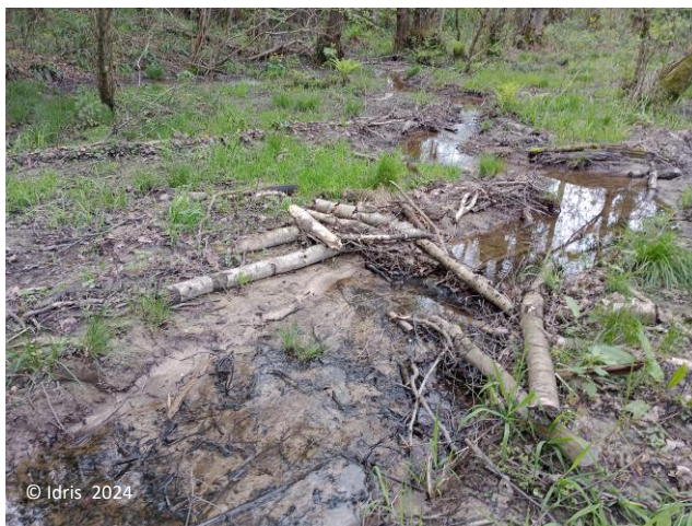
Alder Carr wet woodland restoration through the construction of leaky dams, near Hartfield, West Sussex.
