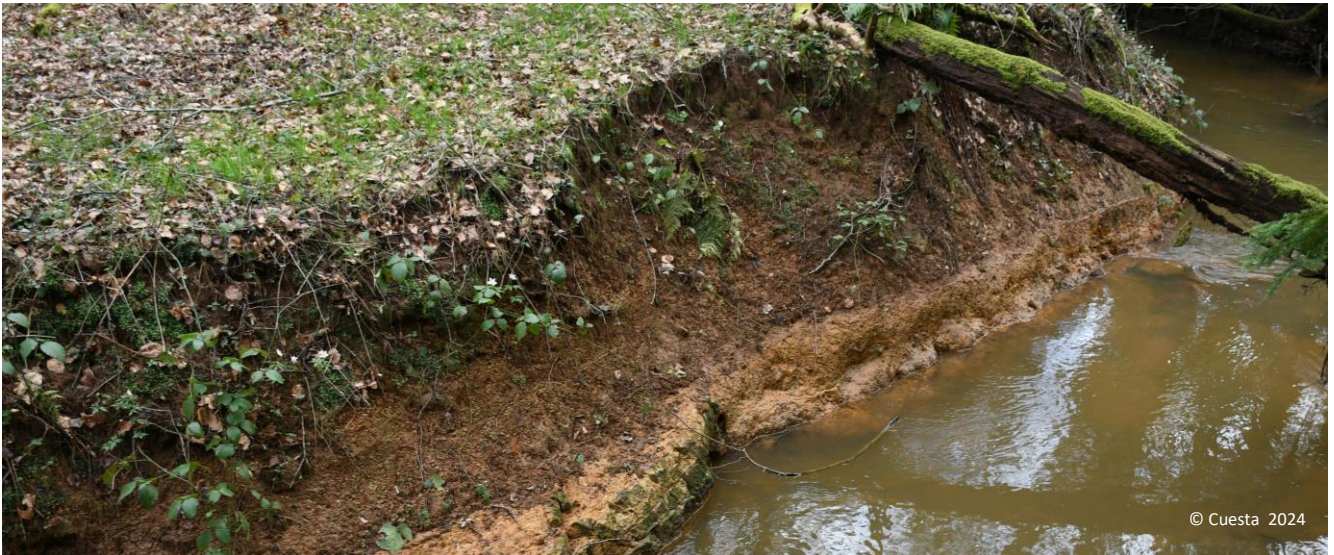
Above: Detail of the cohesive, silty alluvium exposed in the banks of the Shortbridge Stream within the Rock Wood SSSI.
